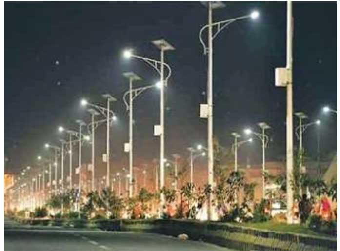
Figure 5-13 Solar Street Lamps (Source: KMC)
